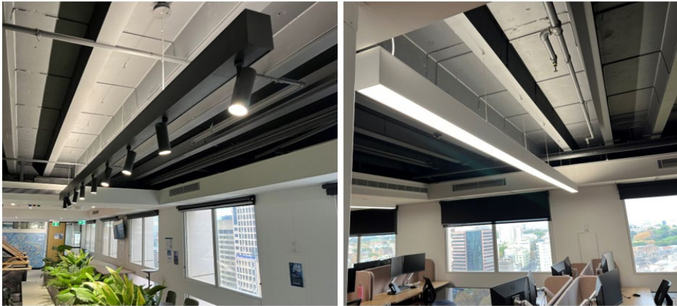
FIGURE 21: LED DOWNLIGHTS (LEFT) AND LED STRIP LIGHT FITTING (RIGHT)
