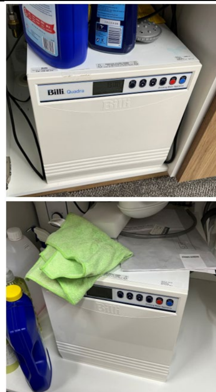
FIGURE 19: UNDER SINK BILLI BOILING, CHILLED WATER UNITS
