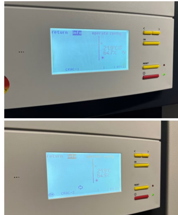
FIGURE 20: DISPLAY ON CRAC UNITS 1 AND 2 INDICATING TEMPERATURE AND RELATIVE HUMIDITY SETPOINTS.
